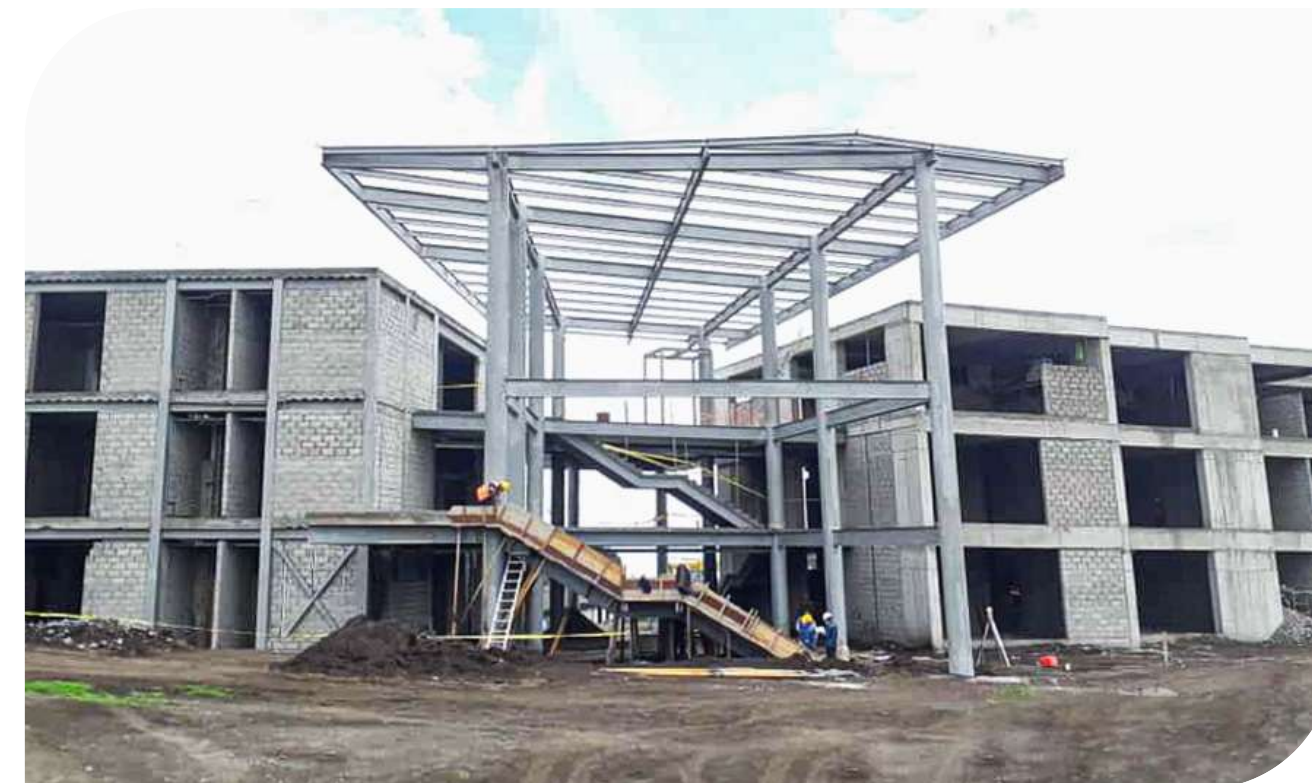
● CONSTRUCTION OF THE TISALEO CAMPUS OF THE UNIVERSIDAD REGIONAL AUTÓNOMA DE LOS ANDES University campus.
