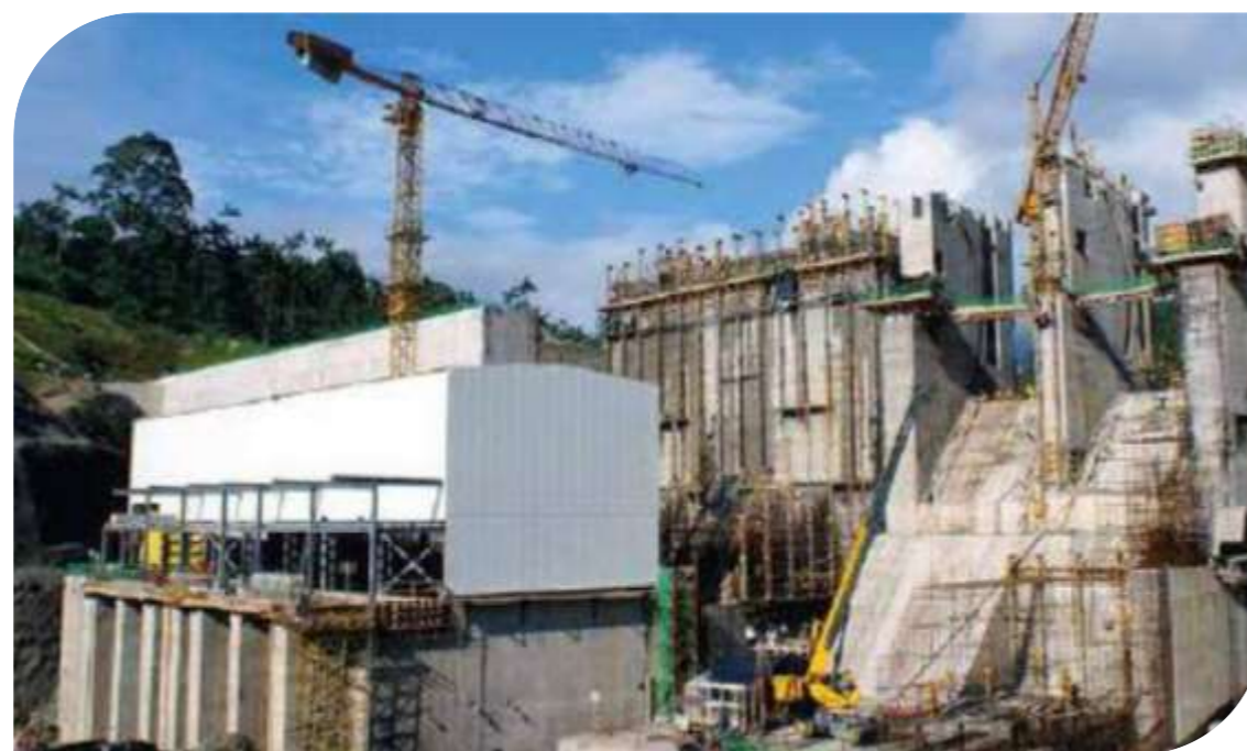
● MANDURIACU Hydroelectric Power Plant.
