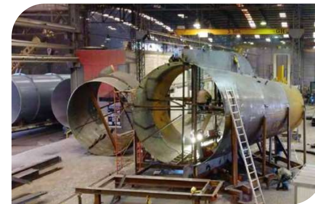
● TOACHI PILATÓN Pipe and Splitter of the Hydroelectric Power Plant.
