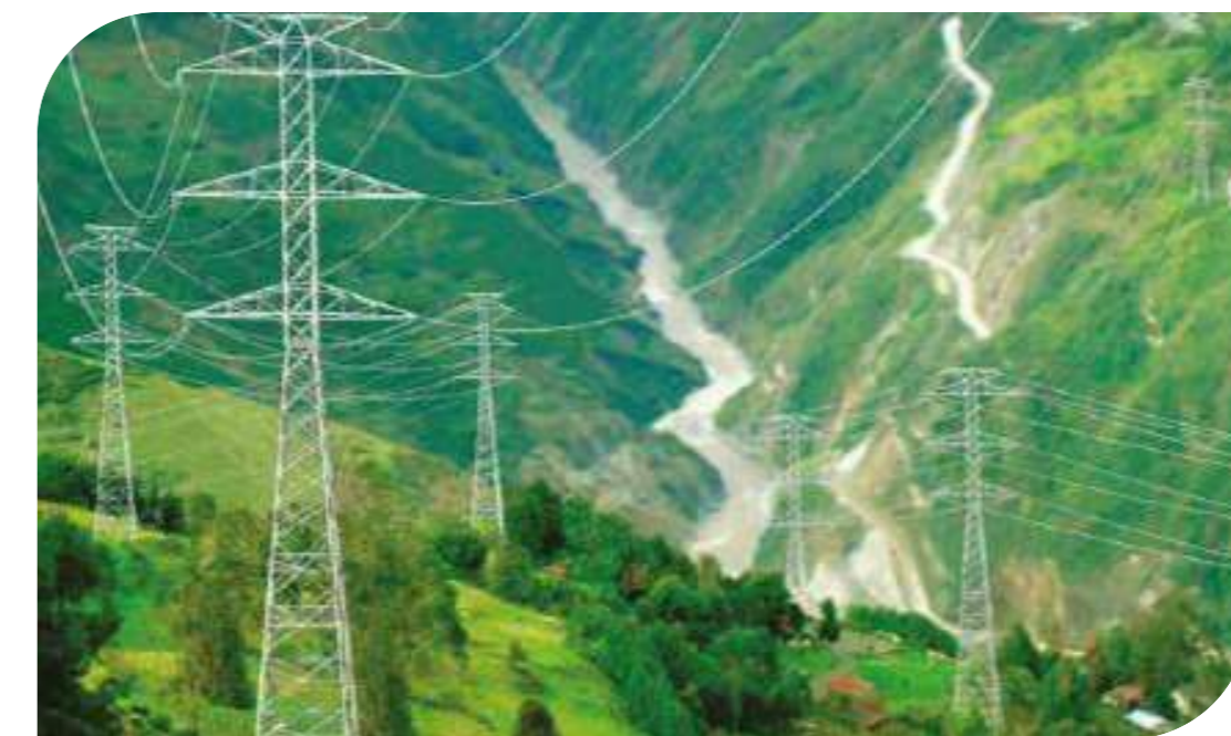
● Mazar- Shoray 220KV Transmission Line.
