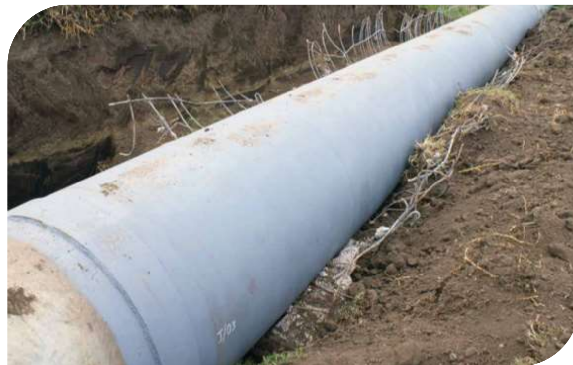
● HYDROELECTRIC PLANT SAN RAFAEL Pipeline
