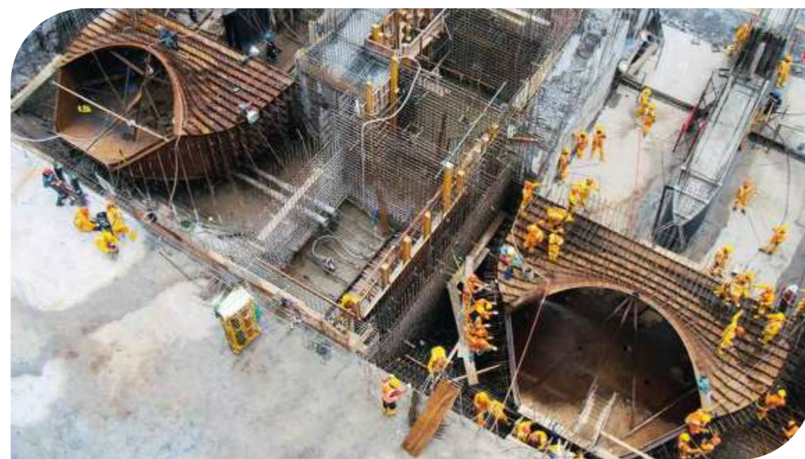
● HIDROELECTRIC PLANT MANDURIACU Suction Elbows
