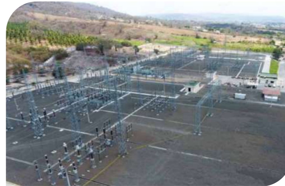
● San Gregorio 230 kV and 69 kV Substation.
