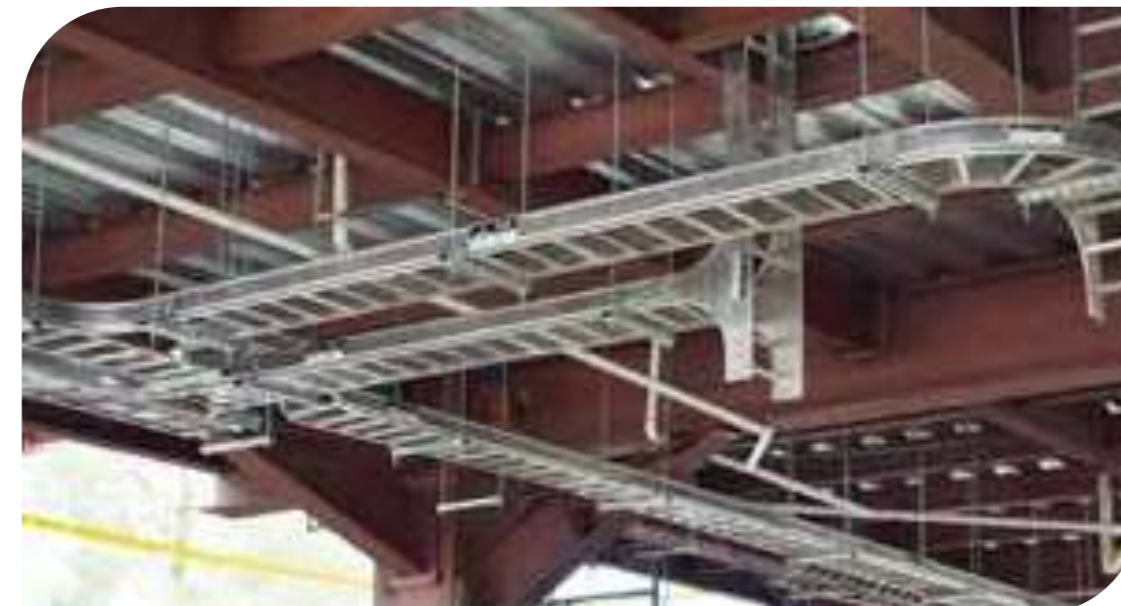
• ESPE Investigation Center 3.500 m of light aluminum trays.
