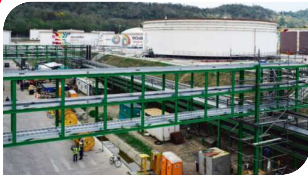
• Repowering of the Esmeraldas Refinery – 15,000 m of trays and 100 TON of tray racks and frames.
