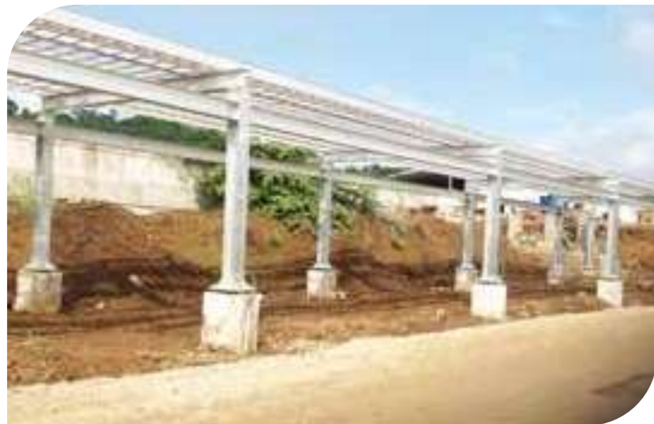
• Chorrillos Monte Verde 8.500 m of heavy aluminum trays and tray rack structures.
