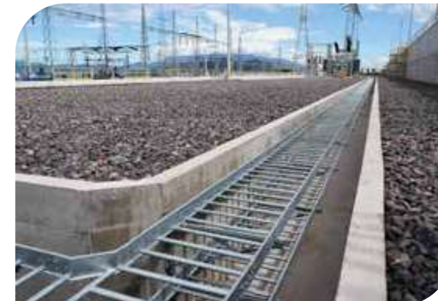
• El Inga Substation 1.200 m of galvanized trays.
