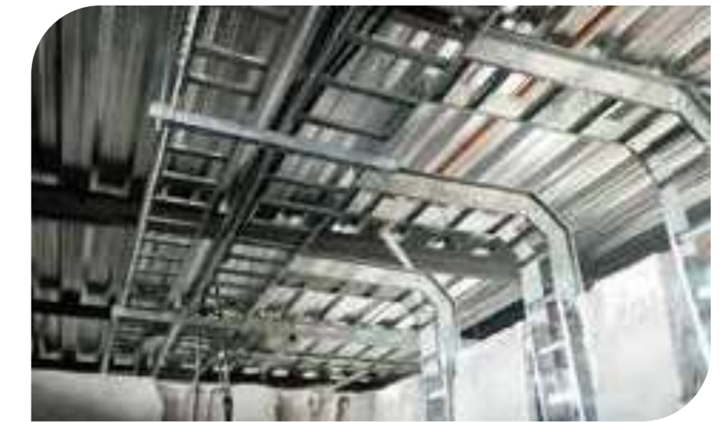
• Coca Airport 500 m of pregalvanized trays.
